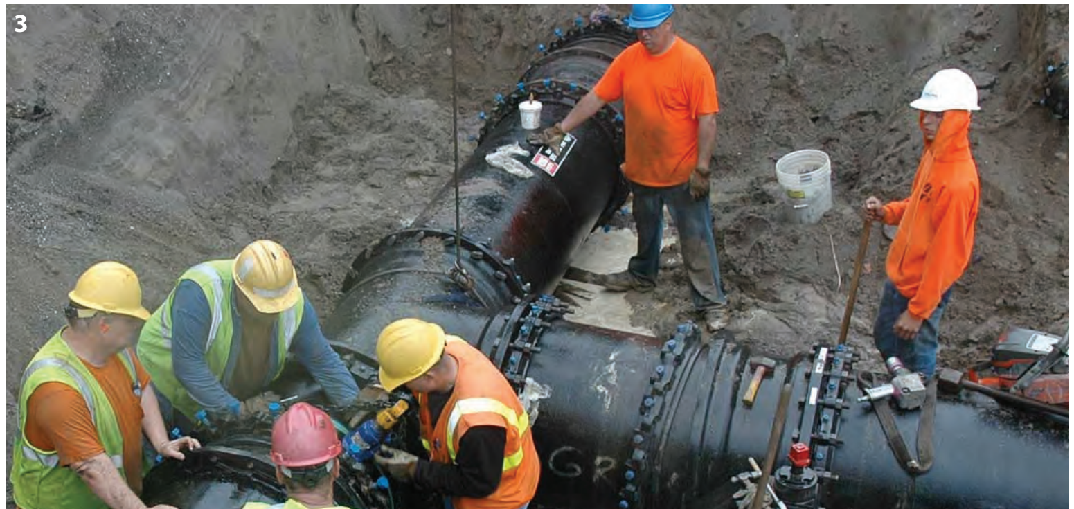
Images: 1. Booster Station Pumps 2. 14th & Grand Tank 3. Installing a T in a Transmission Main
