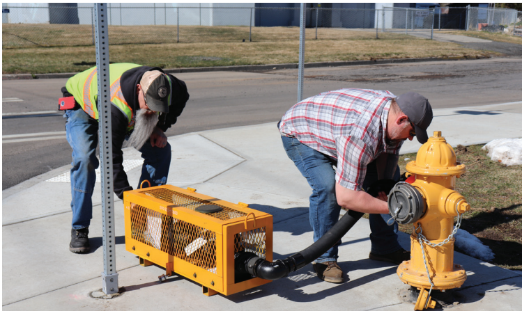
Cross Connection Control Specialists demonstrate proper use of a City hydrant.
