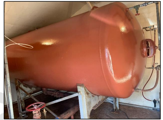
Current Tank Supplying Pressure to Distribution System
