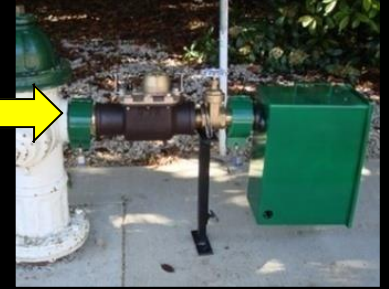
Water Meter Stand
