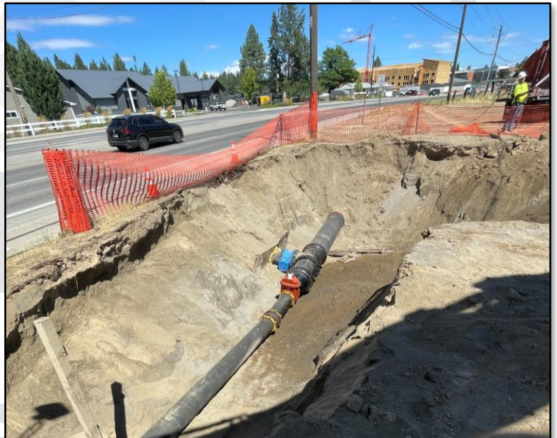
24" x 18" x 12" Connection Point at Hastings Road
